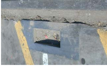
Figure 7. Wharf tiedown bracket failure due to bending
