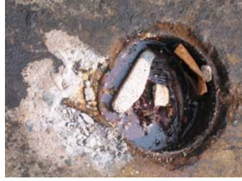
Figure 8. Wharf stowage pin socket failure
