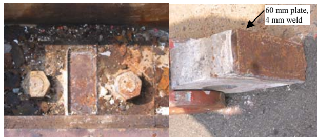
Figure 6. Wharf tiedown bracket failure due to insufficient weld capacity
